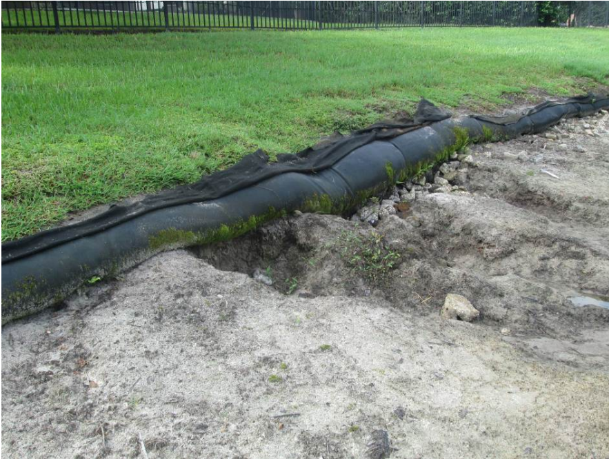
Pond 8 – Exposed & undermined geotube on east side
