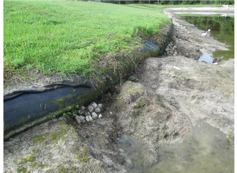
Pond 8 – Exposed & undermined geotube on east side
