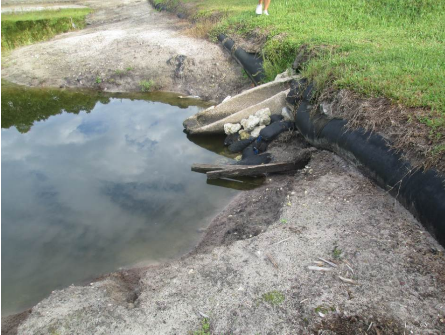
Pond 8 – North side MES undermined
