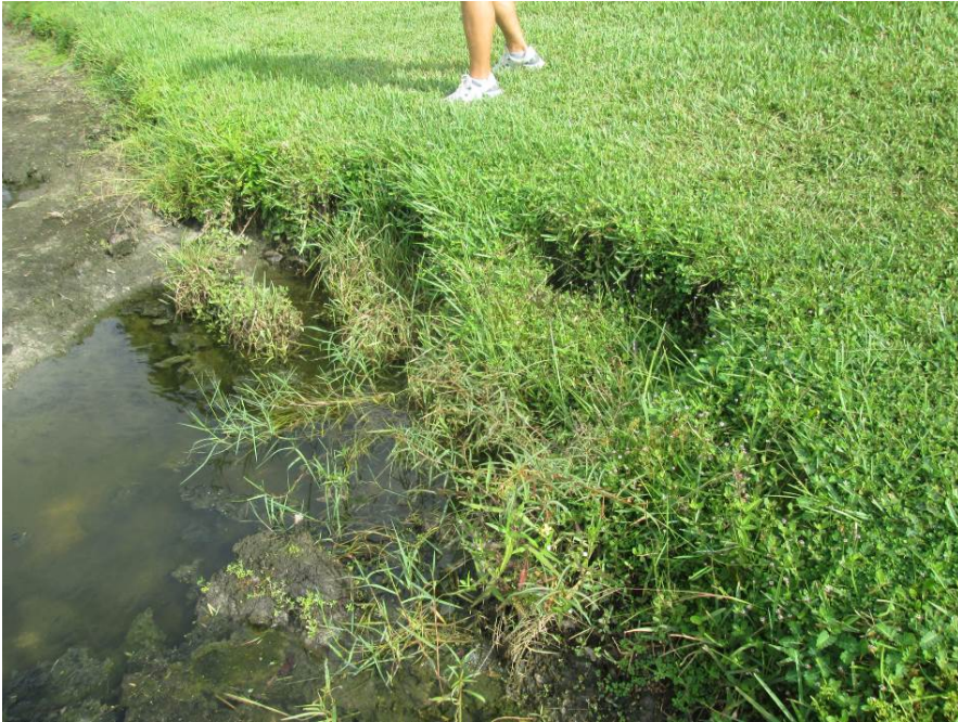
Pond 11 – Point Erosion, possible drain pipe needs to be extended
