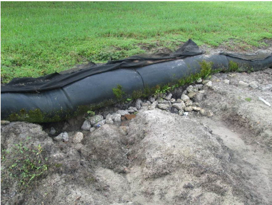
Pond 8 – Exposed & undermined geotube on east side
