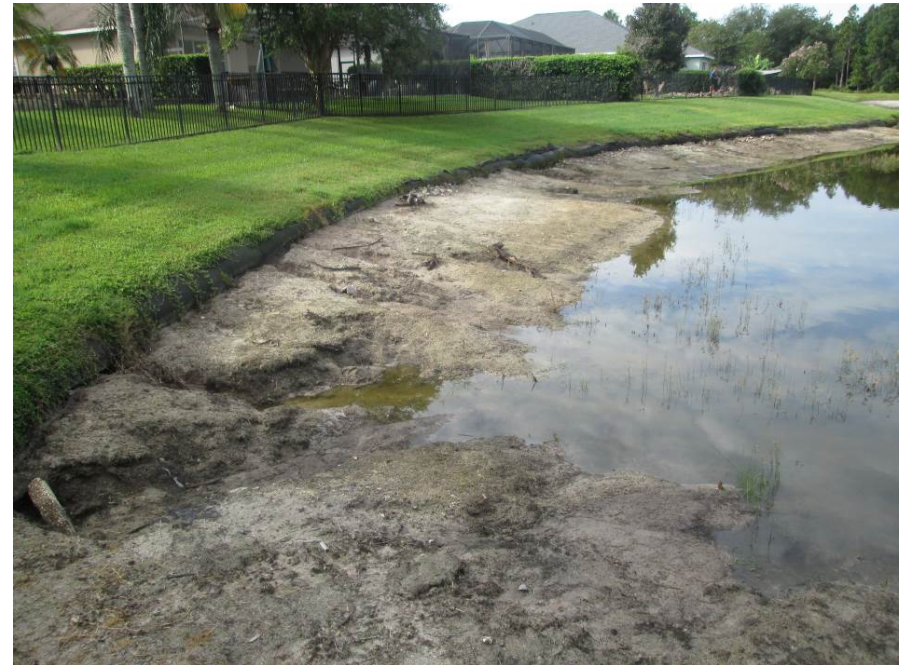
Pond 8 – Exposed & undermined geotube on east side
