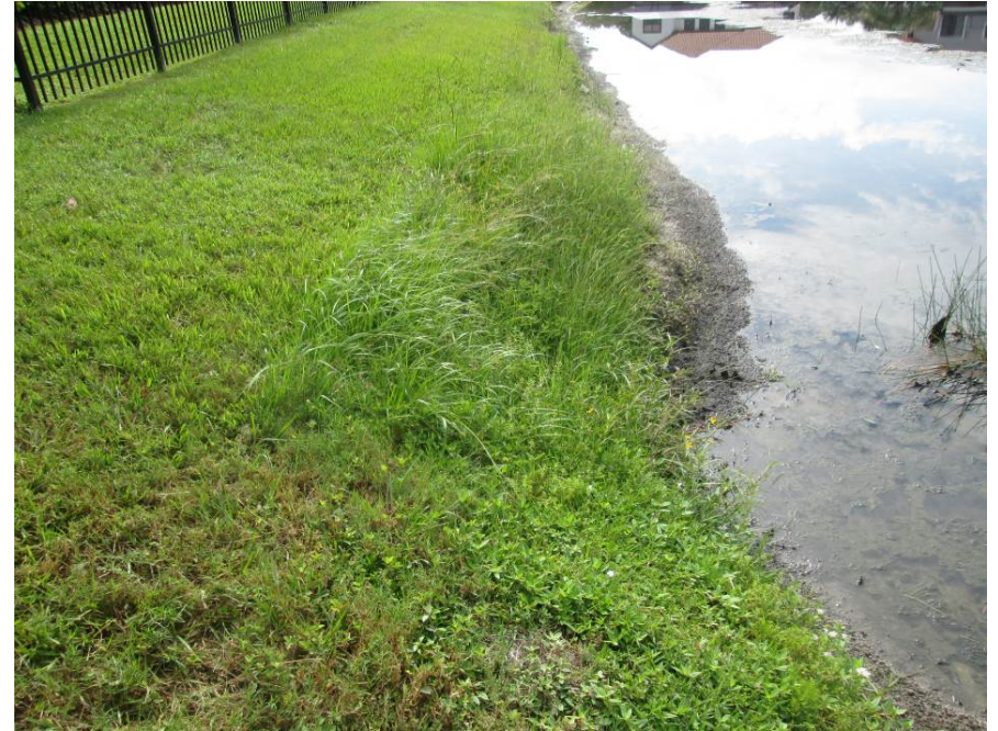
Pond 16 – Minor spot erosion
