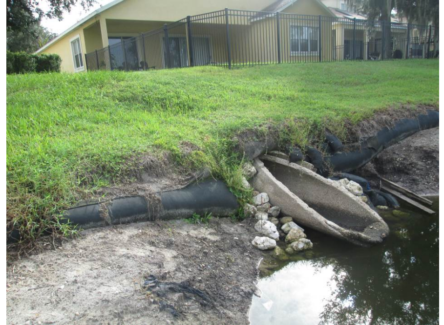
Pond 8 – MES undermined, void above joint
