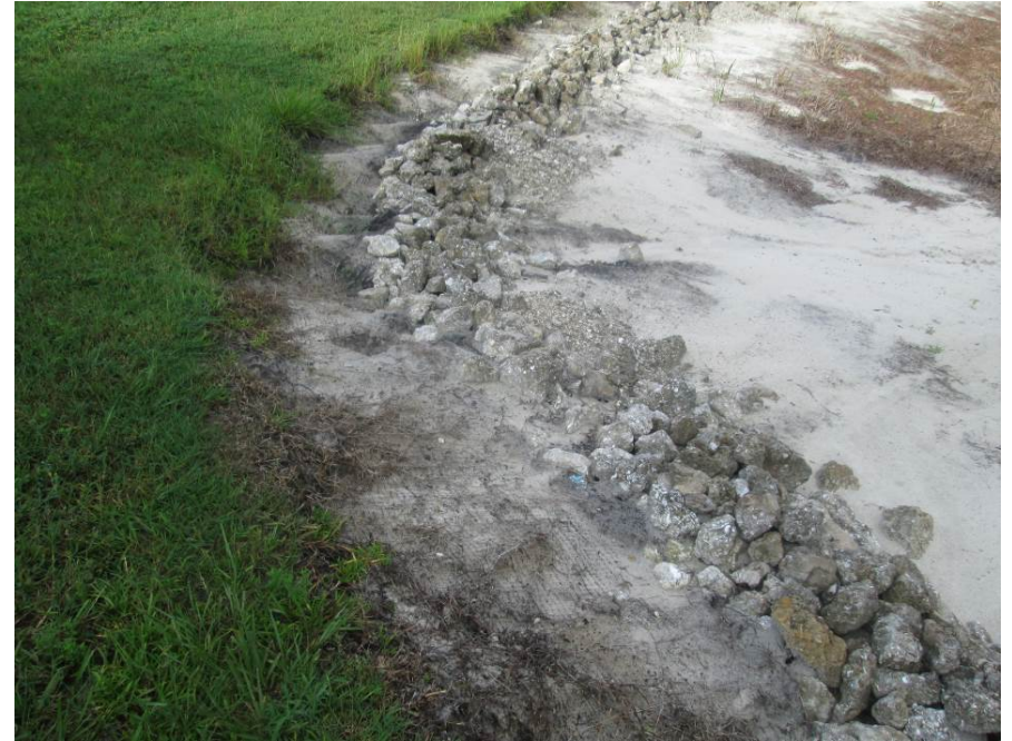
Pond 41 – erosion at control water level, exposed fabric, add fill & rip rap
