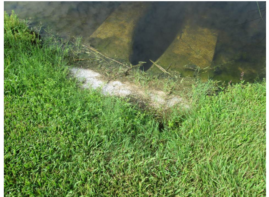
Pond 17 – Void behind MES on north side
