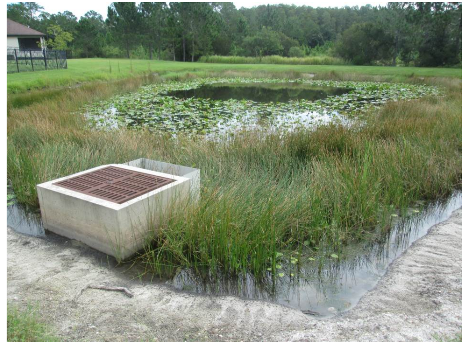
Pond 32 – southwest corner viewing northeast
